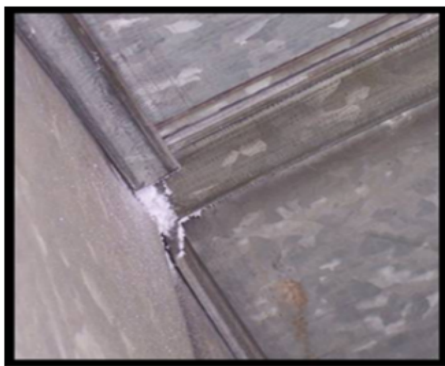
The sealant does not coat the duct interior, but, rather, forms around leaks.
